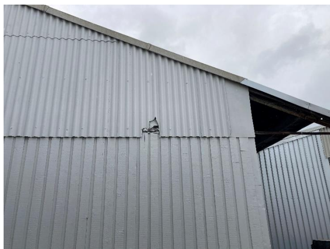
Corrugated fibre cement ('Super-12') cladding on the upper half of the southern end of the building.
