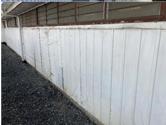
Corrugated fibre cement wall cladding on the southern side of the building.
